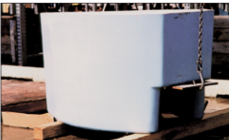
Step 7: After concrete has cured, use hoist plate* / fastout device** and suitable rigging*** to turn basin right-side up
